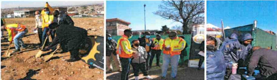
Fig 1: The City of Joburg Mayor Geoff Makhubo and the MMC of Housing Mlungisi Mabaso breaking ground in Alexandra township for the TAC's
